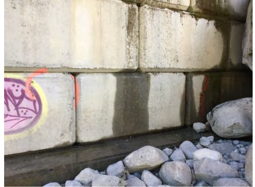
Lock block damage at right abutment
